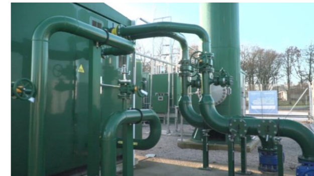
HyDeploy hydrogen gas grid injection into a low pressure network 5
